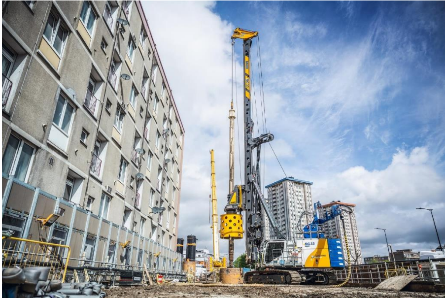
(1) Working on a live project: The BAUER eBG 33 is in operation on an HS2 project in London. © BAUER Group
