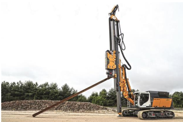
(1) The sheet pile driving assistant is an effective tool for accurate and rapid handling of sheet pile elements.
