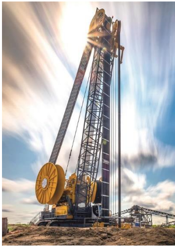
(2) Depth record: In 2019, a depth of 251.4 m was reached for the first time with a Bauer cutter.
