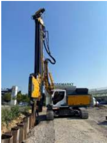
(2) RG 19T with integrated sheet pile assistant at a project in Karlsruhe, Germany
