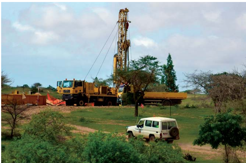
Grand Cote, Diogo, Senegal Installation of 550 m deep mine water supply wells
