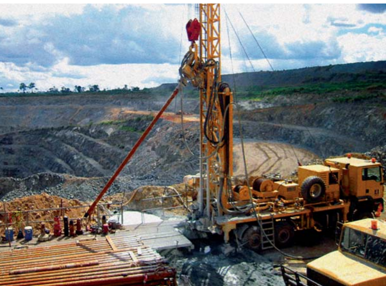
Gold mine, Ghana Dewatering wells for open pit operations
