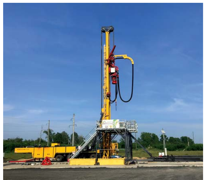
Coal mine, Kuzbass Region, Russia Installation of 550 m deep ventilation shafts of up to 1,500 mm diameter
