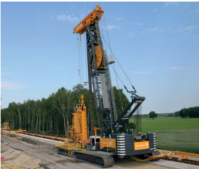
Vattenfall lignite mine, Germany Installation of a 150 m deep clay core cut-off wall with a customized electrically driven cutter system
