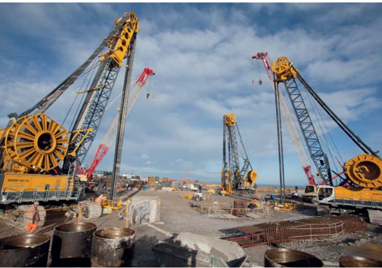
Woodsmith Mine, United Kingdom Construction of circular diaphragm wall shafts up to 35 m diameter
