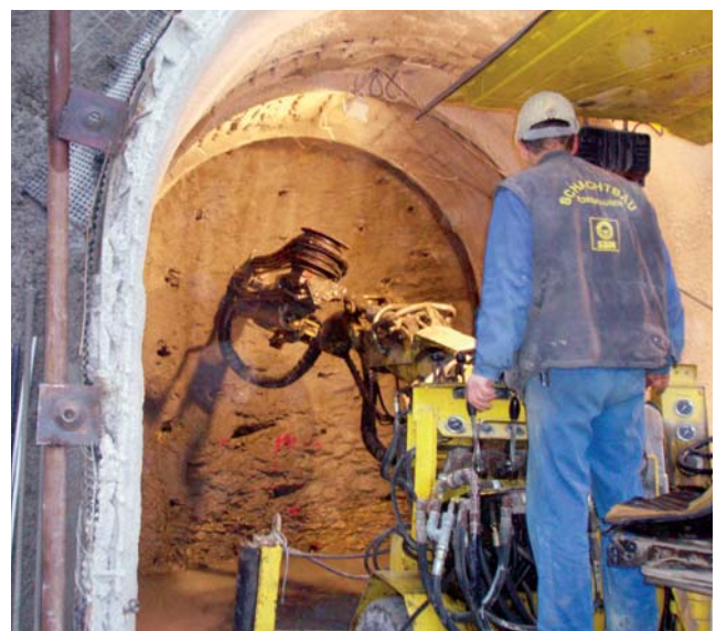
Bleicherode, Germany Conventional drifting with drilling and blasting in a heap adit
