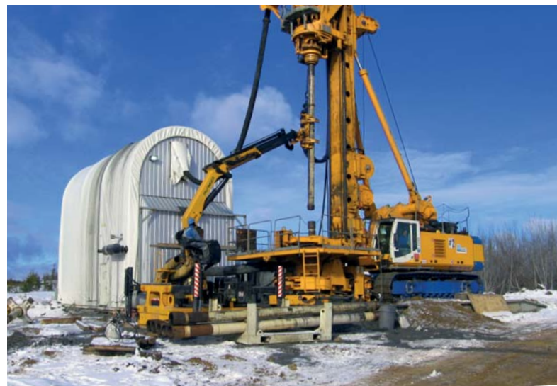
Shore Gold Inc., Saskatchewan, Canada Kimberlite bulk sampling, dia.1.2 m with RC system on BG up to 360 m depth
