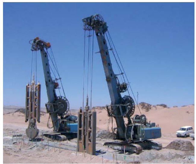
Namdeb Mine, Pocket Beaches, Namibia Cement bentonite cut-off wall along the Atlantic Ocean for alluvial open pit mining
