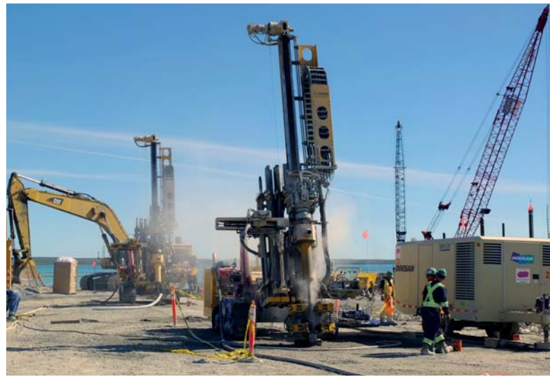
Diavik Diamond Mine, Northwest Territories, Canada Curtain grouting and jet grouting on dike A21
