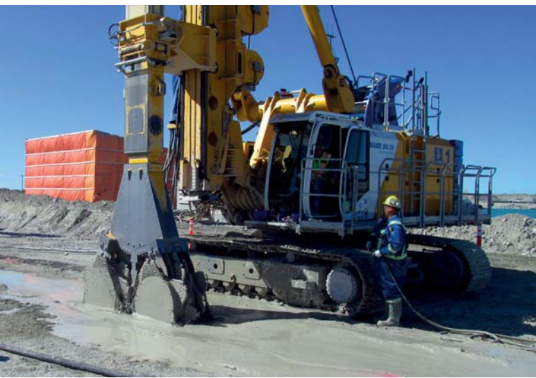
Diavik Diamond Mine, Northwest Territories, Canada Installation of a cutter soil mixing wall
